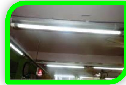
Energy Efficient Lighting
